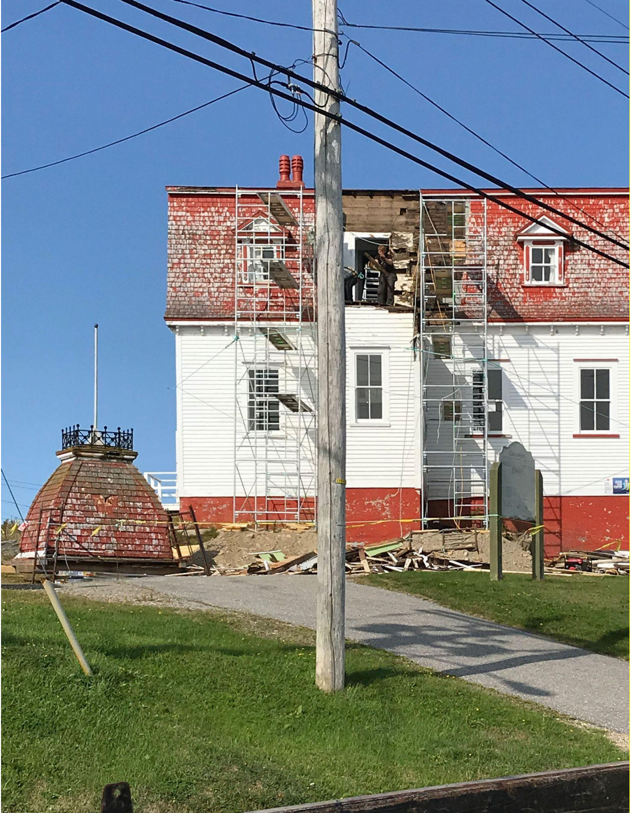
At work restoring the tower and cupola of the historic Greenspond Courthouse.
