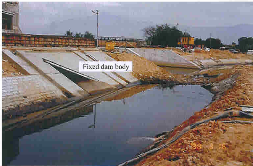
Fig. 1. Water flowing over fixed rubber dam body.
