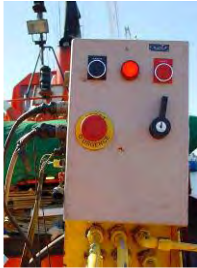
GAMBAS® 50 Safety Devices – Circuit Breaker on the Control Panel
