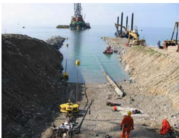
Figure 4-7 Shore Crossing with Pipeline Pulled to Shore via Onshore Sheave (Bluestream, Russia)
