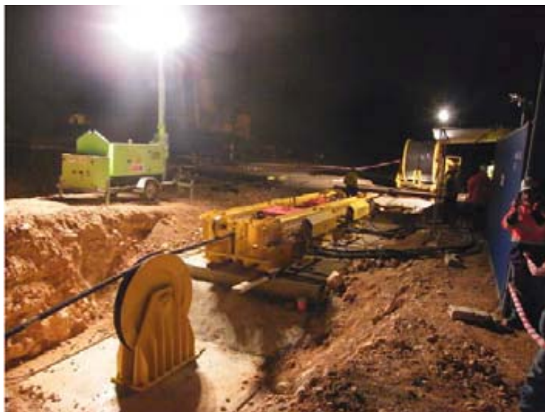
Figure 4-5 Shore Crossing with Pipeline Pulled to Shore with linear Winch (Ibiza, Spain)
