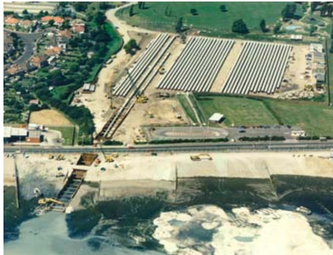
Figure 4-8 Shore Crossing with Pipeline Assembled on Shore and Pulled into Sea with Pulling Barge
