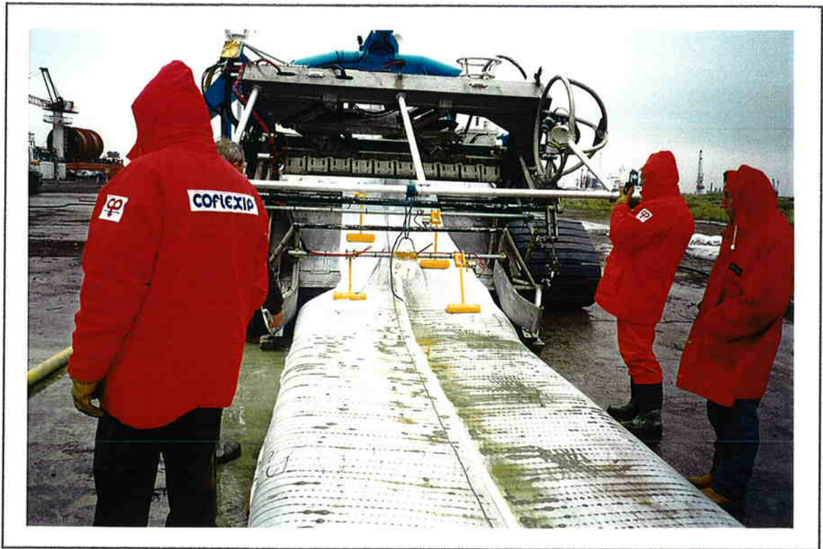
Accurate follow up of the cable to be protected by the laid mattress
