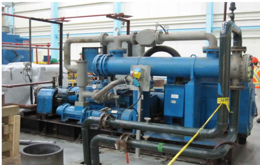
Figure 1 Photograph of unit 3 acceleration skid PGC model HL60/9HS
