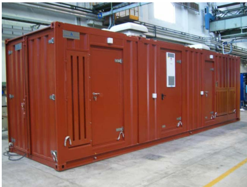
Figure 10 Typical Static Start Unit from [redacted] (note this unit is containerized)
