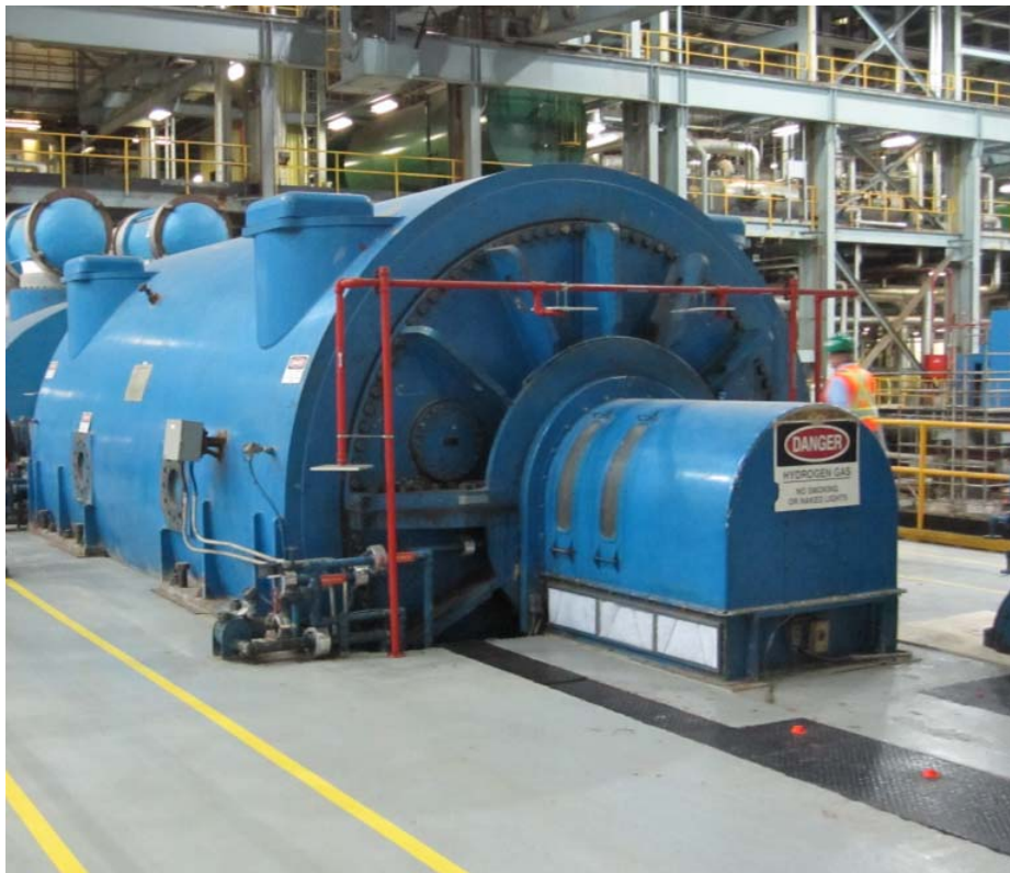
Figure 11 Exciter housing, rear of generator, unit 2
