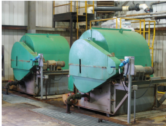
FIGURE 8-24 UNIT 1 CIRCULATING WATER TRAVELLING SCREENS
