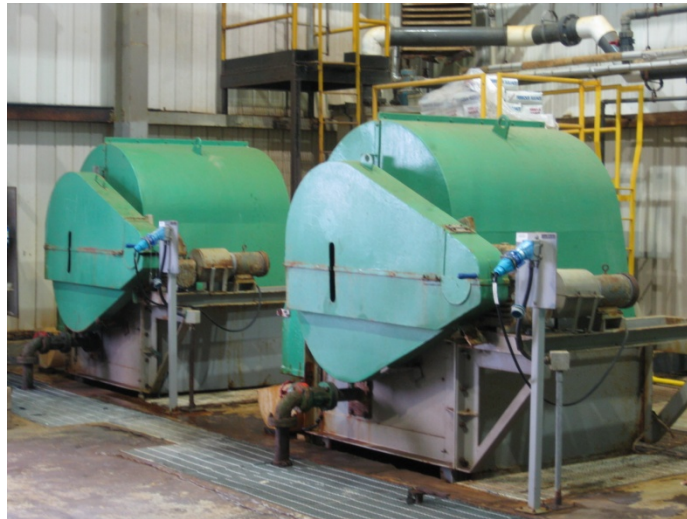
FIGURE 9-25 UNIT 1 & 2 CIRCULATING WATER TRAVELLING SCREENS
