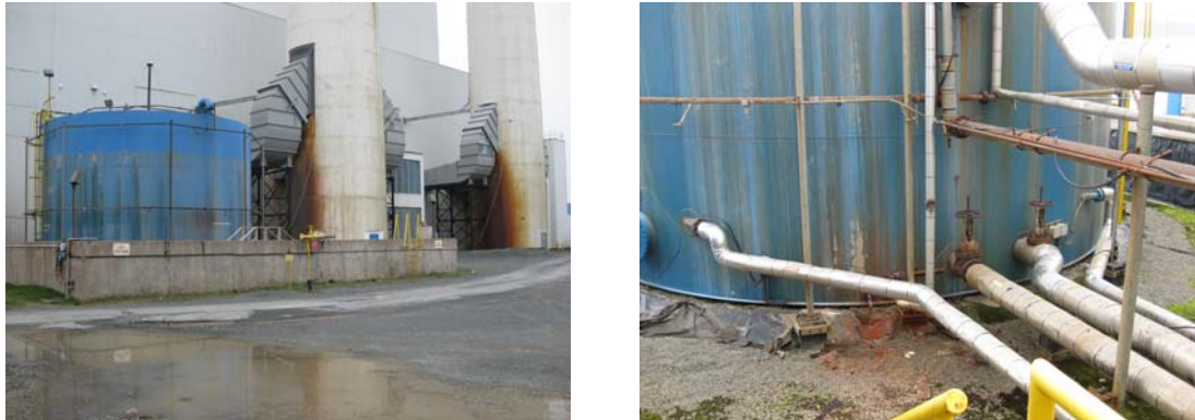
FIGURE 11-24 HEAVY OIL DAY TANK AND PIPING TO POWERHOUSE
