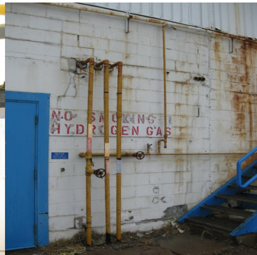
FIGURE 11-18 HYDROGEN LINES INTO POWERHOUSE
