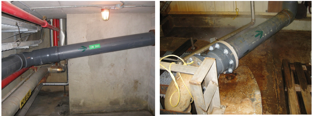
FIGURE 8-8 DEDICATED SEAWATER COOLING WATER LINE FOR UNIT 3 SYNCHRONOUS CONDENSING TG AUXILIARY COOLING WATER
