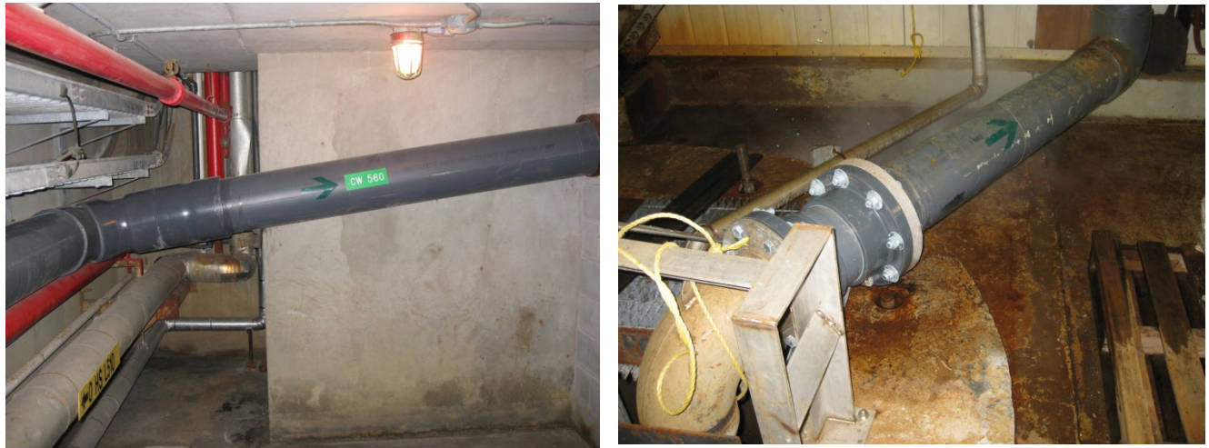
FIGURE 10-11 DEDICATED SEAWATER COOLING WATER LINE FOR UNIT 3 SYNCHRONOUS CONDENSING GT AUXILIARY COOLING WATER
