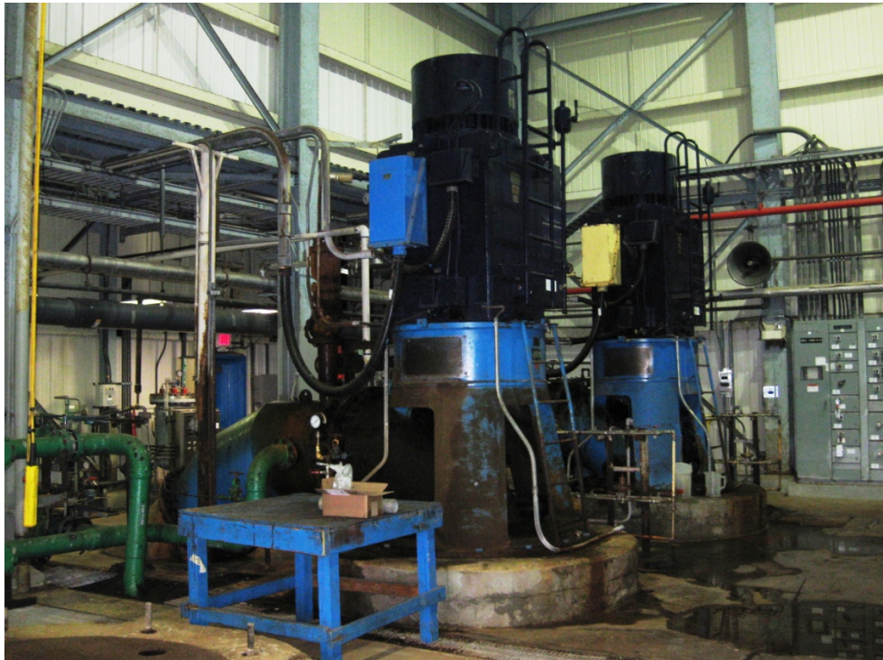
FIGURE 10-28 UNIT 3 CIRCULATING WATER PUMPS
