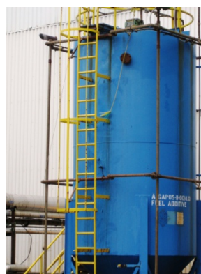
FIGURE 11-25 FUEL ADDITIVE STORAGE TANK
