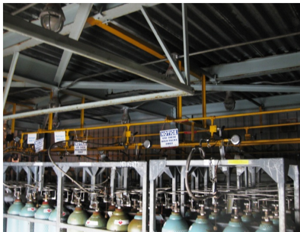
FIGURE 11-15 HYDROGEN STORAGE RACKS
