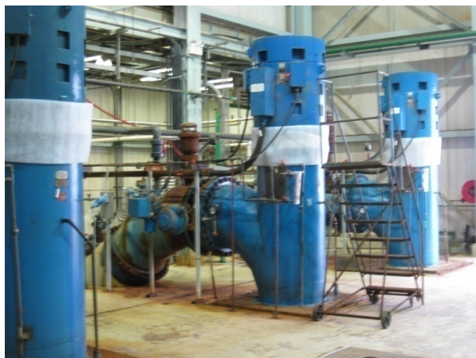
FIGURE 8-23 UNIT 1 CIRCULATING WATER PUMPS
