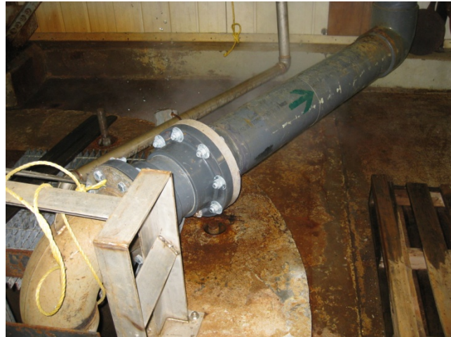
FIGURE 9-8 DEDICATED SEAWATER COOLING WATER LINE FOR UNIT 3 SYNCHRONOUS CONDENSING GT AUXILIARY COOLING WATER
