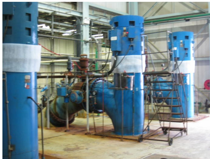
FIGURE 9-24 UNIT 1 & 2 CIRCULATING WATER PUMPS
