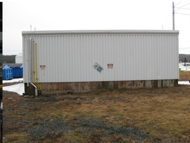
FIGURE 11-16 HYDROGEN STORAGE BUILDING
