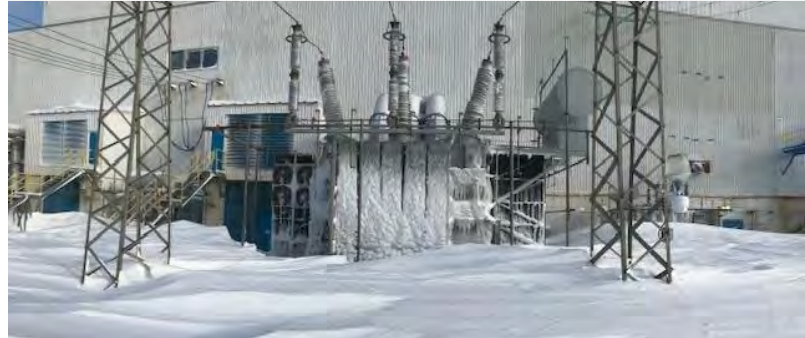
Due to the extreme volume of snow that fell during the blizzard, electrical equipment at many sites—like the transformer shown above in Holyrood—quickly became covered in snow.
