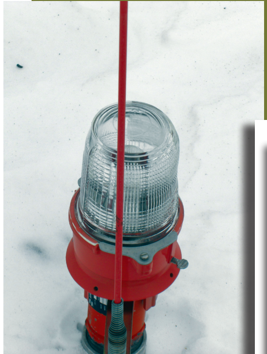
Airstrip Runway Edge Lighting
