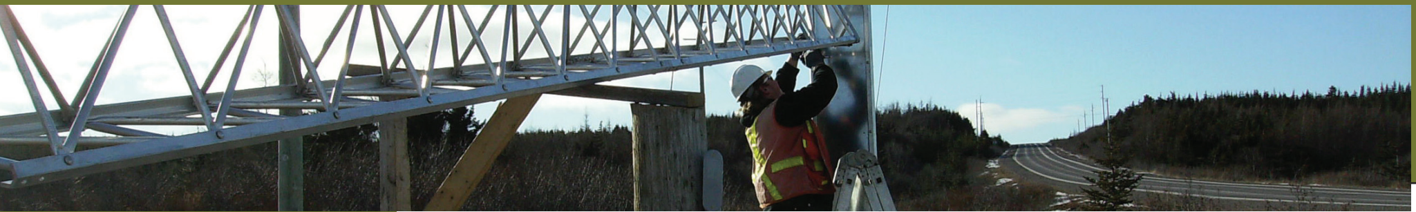
Intelligent Transportation System - Grand Bank Installation
