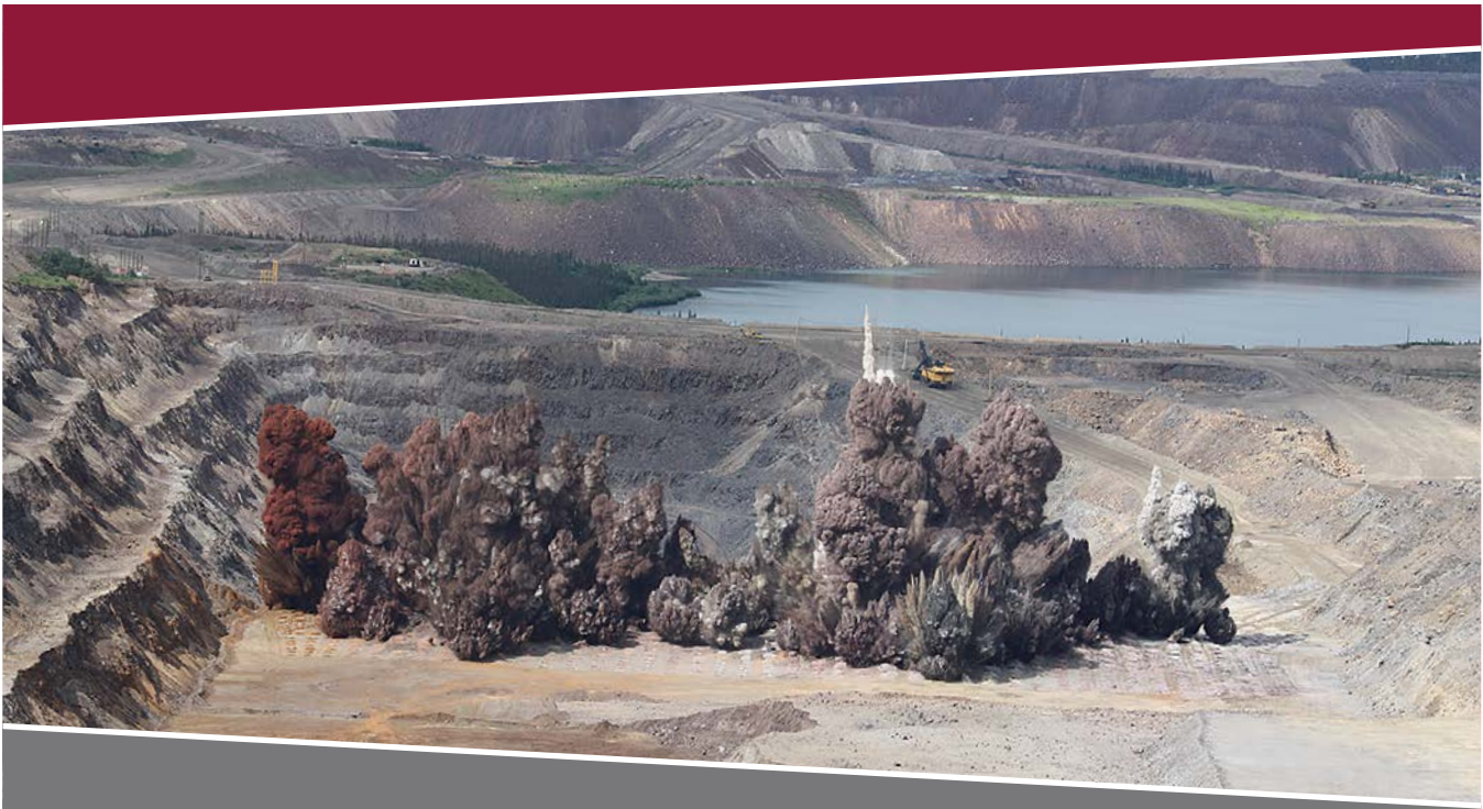
Blasting operations at IOC's Luce Pit, Labrador City. Courtesy: Iron Ore Company of Canada.
