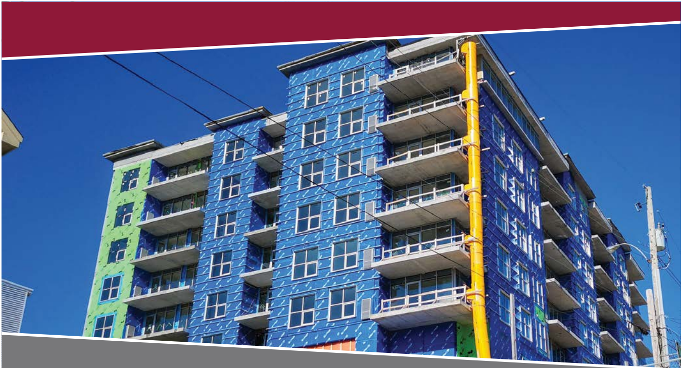
Star of the Sea Residences, Henry Street, St. John's. Courtesy: Department of Finance.
