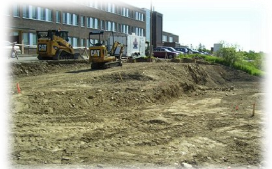
Construction begins on therapeutic garden at James Paton Memorial Regional Health Centre
