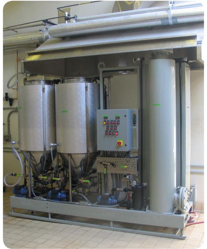
MI Biodiesel Project
