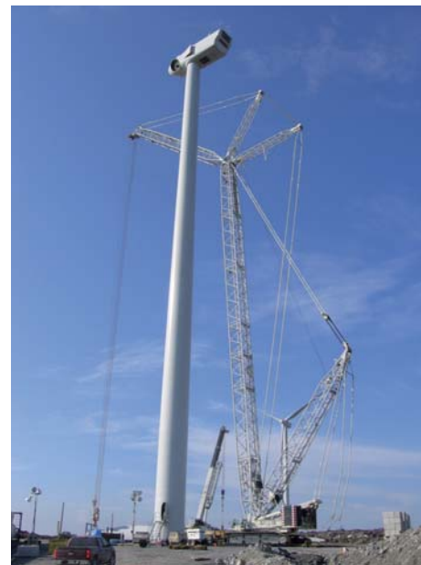
Fermeuse Wind Farm. Photo P.Carter.
