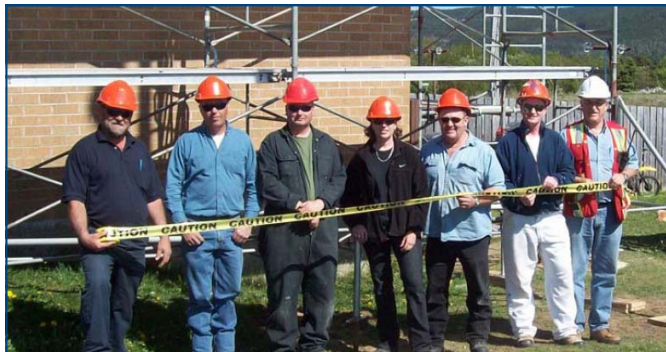
NL Housing's Avalon Regional Office Modernization Crew pose next to the newly erected scaffold after the new training certification.
