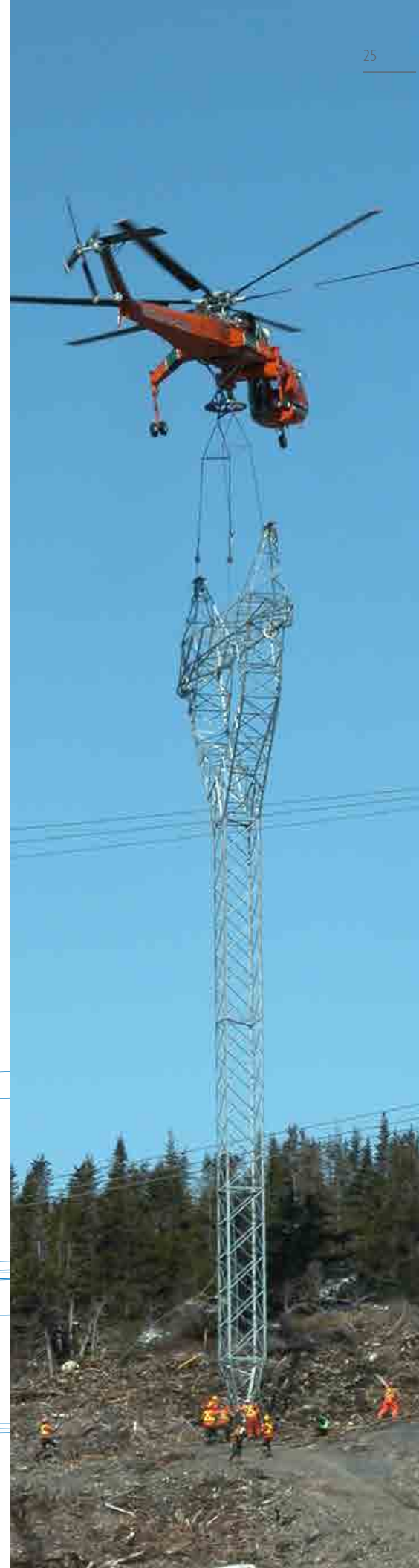
Tower installation, new transmission line from Bay d'Espoir to the Avalon Peninsula
