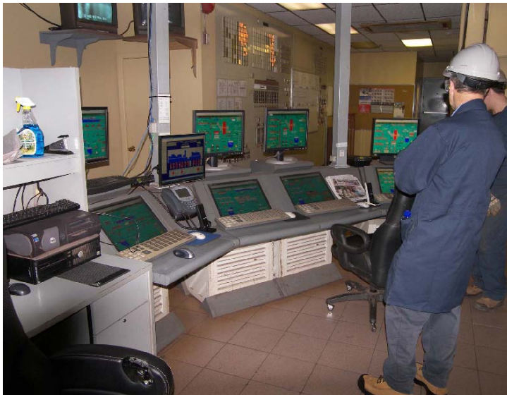
Photo: Control Room at IOC's iron ore Concentrator, Labrador City
