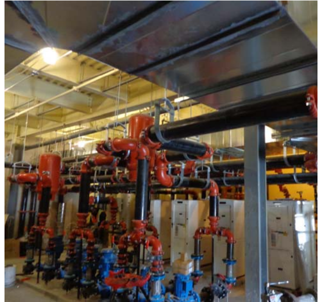
Geothermal Cooling Tower – New Davis Elementary
